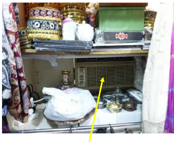
First air conditioner of Baku factory in a souvenir shop in the Old City ("Icheri Sheher")
